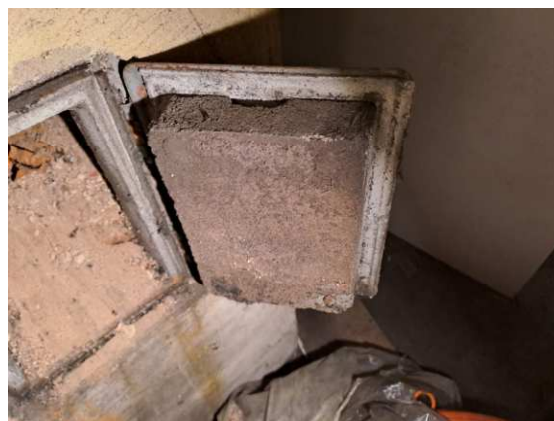
Asbestpappen-Befund in AG 253
